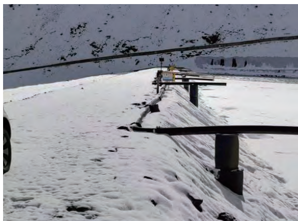
Figure 12.3: Tailings discharge pipe at the dam crest
