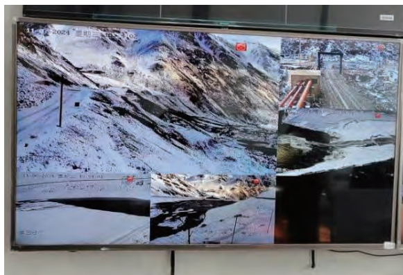
Figure 12.2: Site video surveillance equipment
